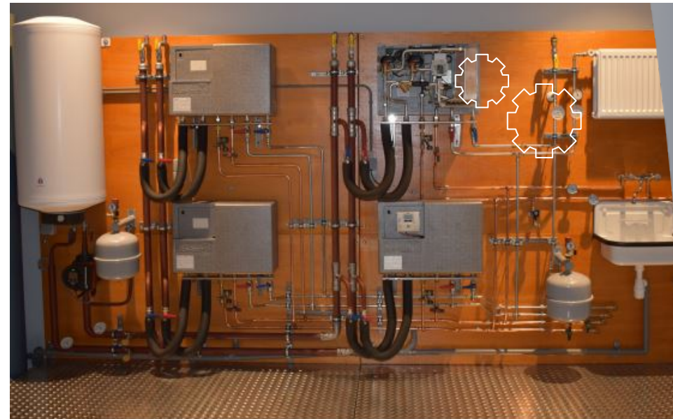
Test & Experience center Que-tech
